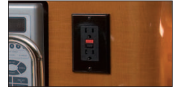
GFI POWER OUTLET
